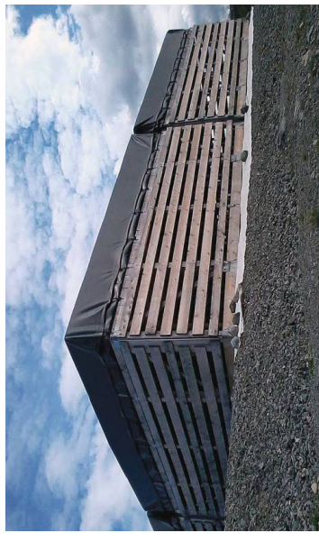
Fig. 3. HBA tile antennas (#83 and #96) on the timber framesets. The material at the base of the frameset is a strip of geotextile, used to prevent erosion along the array edges and between the tiles.
