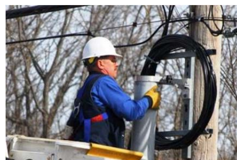
A Sho-Me Technologies construction worker strings fiber that helped increase broadband availability to rural farmers.
